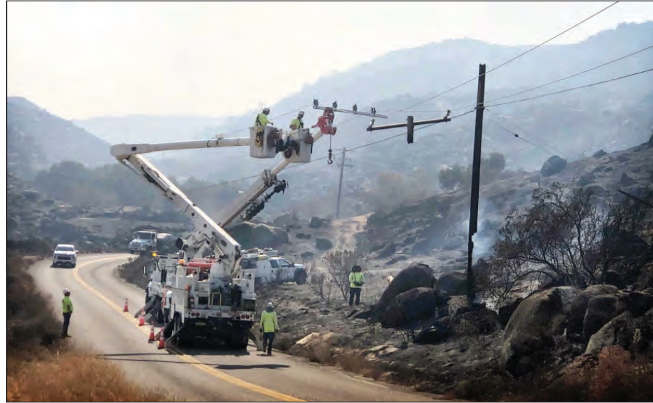
Crews on Sept. 6, 2022, prepare to replace a blackened electrical pole that burned during the Fairview fire near Hemet. | Courtesy Photo of Brian Rokos, The Press-Enterprise/SCNC
